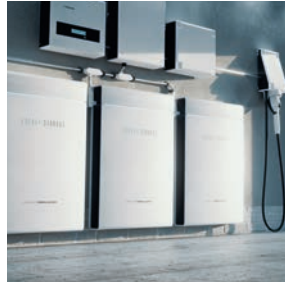
Grid Energy Storage
